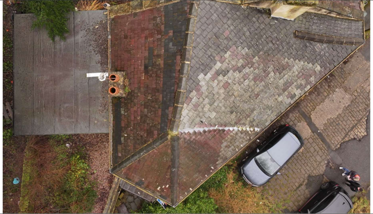
Overhead photo of the roof pitches, the front is to the right-hand side of the photo.
